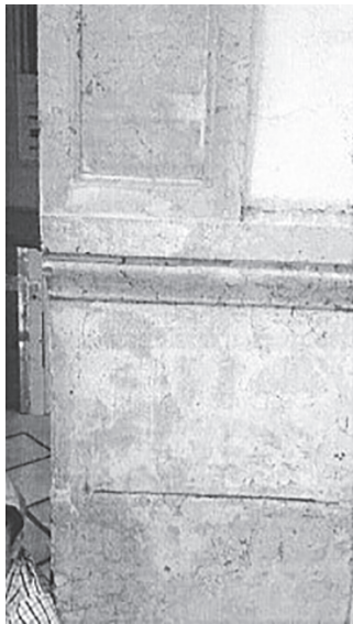
Figure 1. Color changes in the restoration material used in natural stone cracks on a facade (photo by Olga Smirnova in Malaga city center in 2019)
