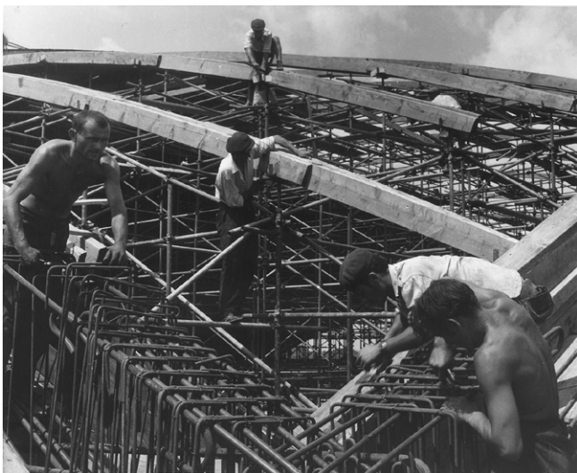
Figure 7. Construction of Hall 2 of the Belgrade Fair – assembly of the rebar for the edge arches and the structure of the shell (Source: https://sajam.rs/en/sanu-exhibition-dedicated-to-the-belgrade-fair-phenomenon-on-local-and-global-scale/# )
