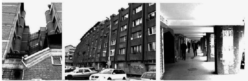
Figure 8. Old Lučna building: outlook, side view showing double tract, back of buildings and shopping street
